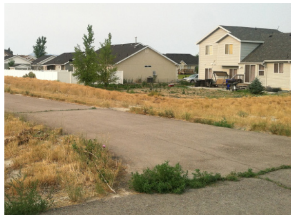
Cracks in asphalt shared-use paths can allow weeds and grasses to grow up, worsening the crack and blocking use of the path
