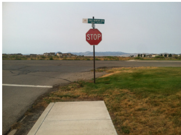
Sidewalk gap at an Eagle Mountain Blvd intersection in City Center
